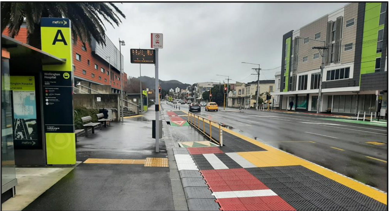
Figure 2 Zicla bus stop being installed outside the hospital for the Newtown to City Transitional Cycleway
