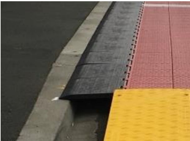
Figure 6: Footpath ramp lacking slip resistance (black units)
